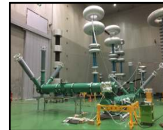
[Bus charging current test]
