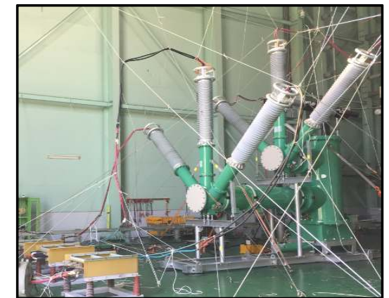
[Short-Circuit test in KERI]
